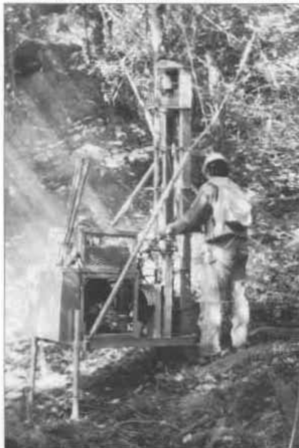
Shallow seismic shot hole drilled as part of the Northwest Natural Gas Company 3-D seismic program at the Mist Gas Field during 1996. The seismic data will be used to develop more underground storage for natural gas.
